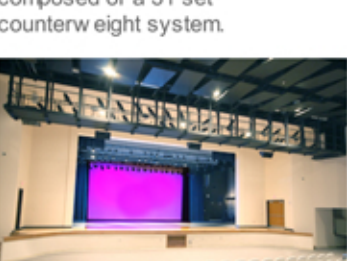
The new lighting system installed by Pittsburgh Stage included traditional lamp fixtures, and variable color LED fixtures.
