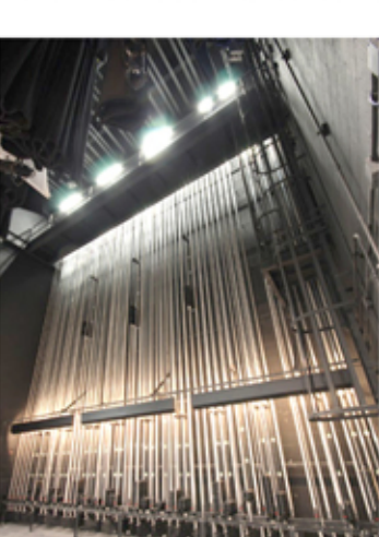
The West Mifflin rigging design is composed of a 31 set counterweight system.
